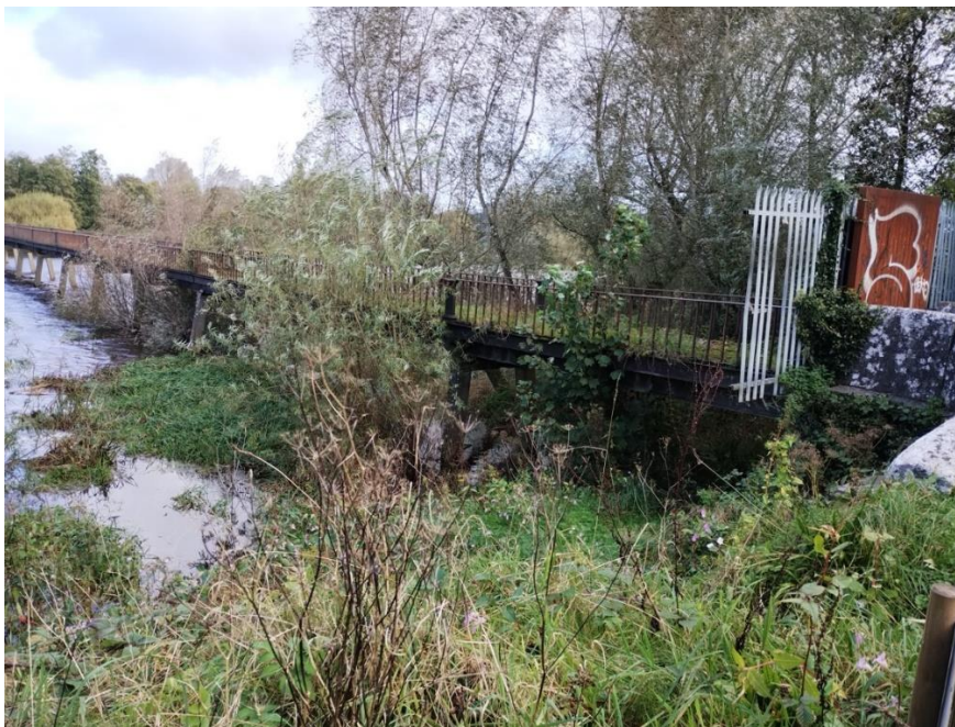
Fig 6 The Black Bridge has been closed for the last five years and is now deteriorating.
